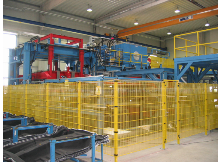
Molding plant – side view
